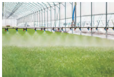
Agricultural greenhouse water supply system
